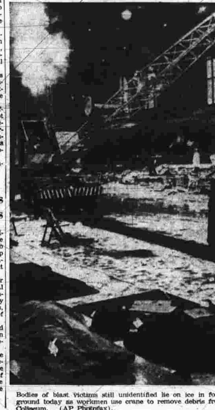
Bodies of blast victims still unidentified lie on ice in foreground today as workmen use crane to remove debris from Coliseum. (AP Photofax).
